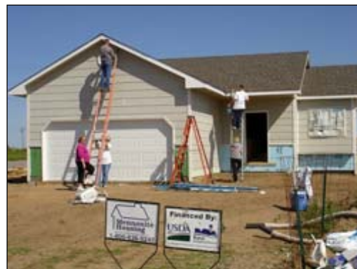
USDA Rural Development volunteers assisted self-help homeowners and Mennonite Housing Rehabilitation Services Inc. staff with caulking, painting, and building interior stud walls for families participating in the Greensburg Community Self-Help Housing Program.
