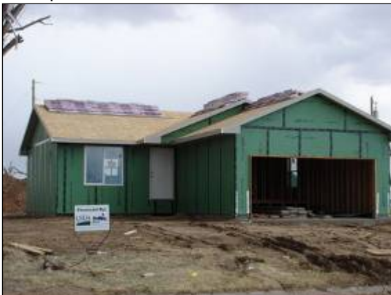
Mennonite Housing Rehabilitation Services, Inc. of Wichita, a faith-based organization has received Technical Assistance Funding from USDA Rural Development to supervise construction of the Agency’s Mutual Self-Help Housing Program . and over the past tens years has been involved in the building of one hundred ten homes, expanding affordable homeownership.
